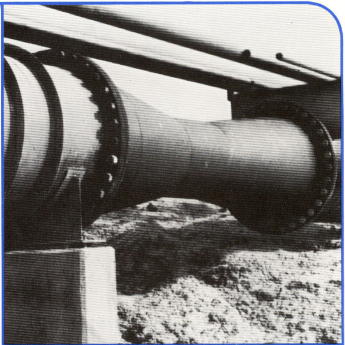
Pictured above is a 36 inch Energy Flow Model VTF Venturi at a large secondary waste treatment facility.
